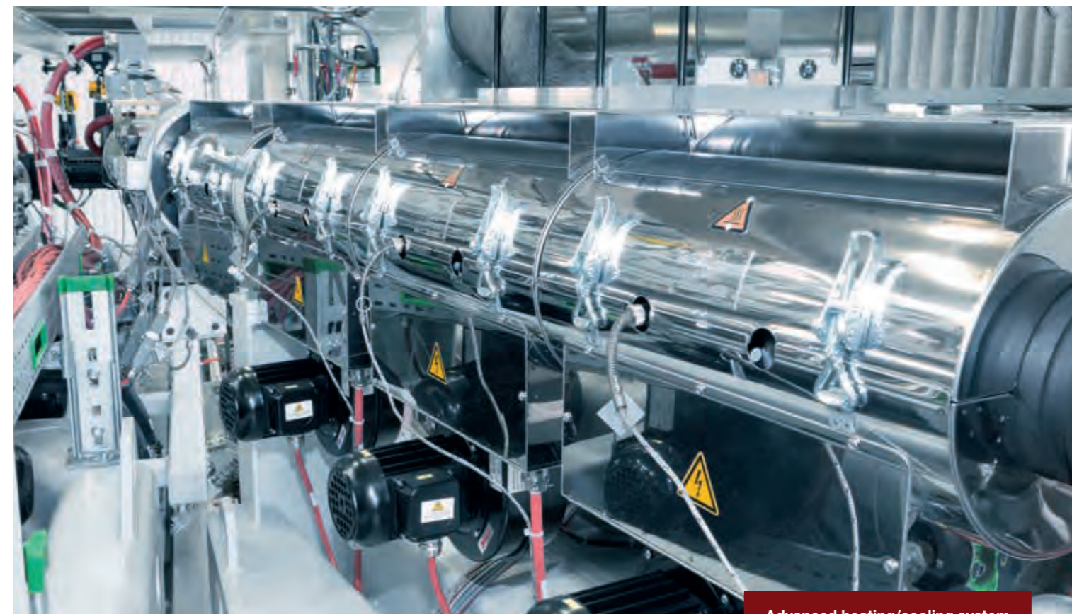
Advanced heating/cooling system
